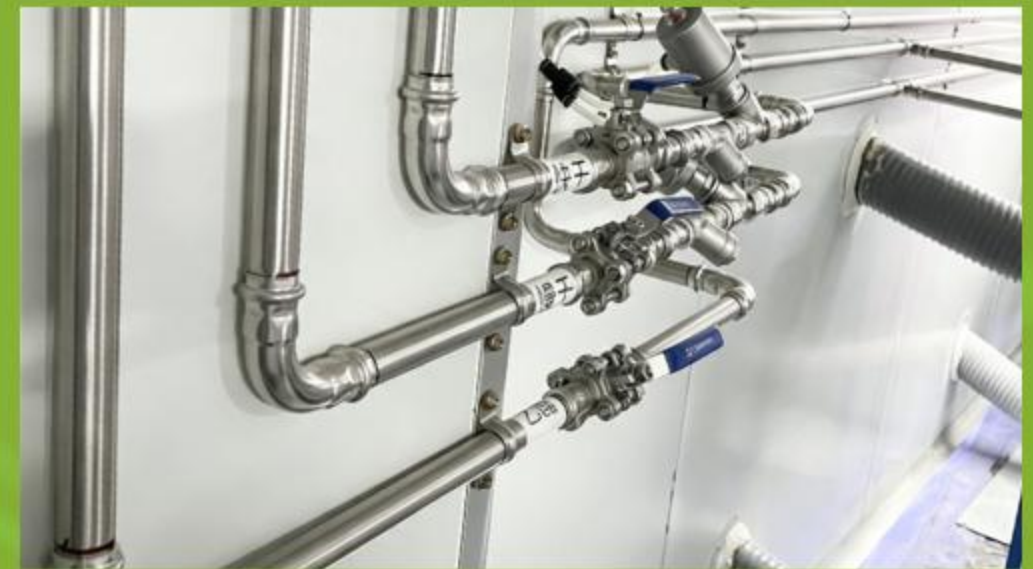
Automatic solvent control system
