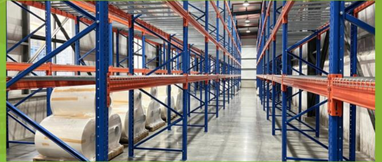
Sprinkler-protected high-bay warehouse
