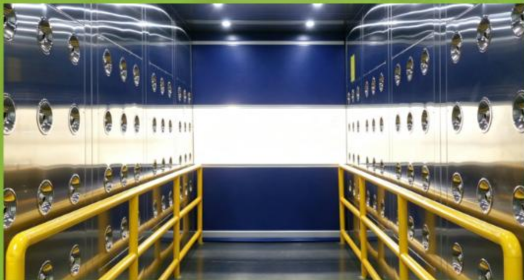
Material air-shower passage
