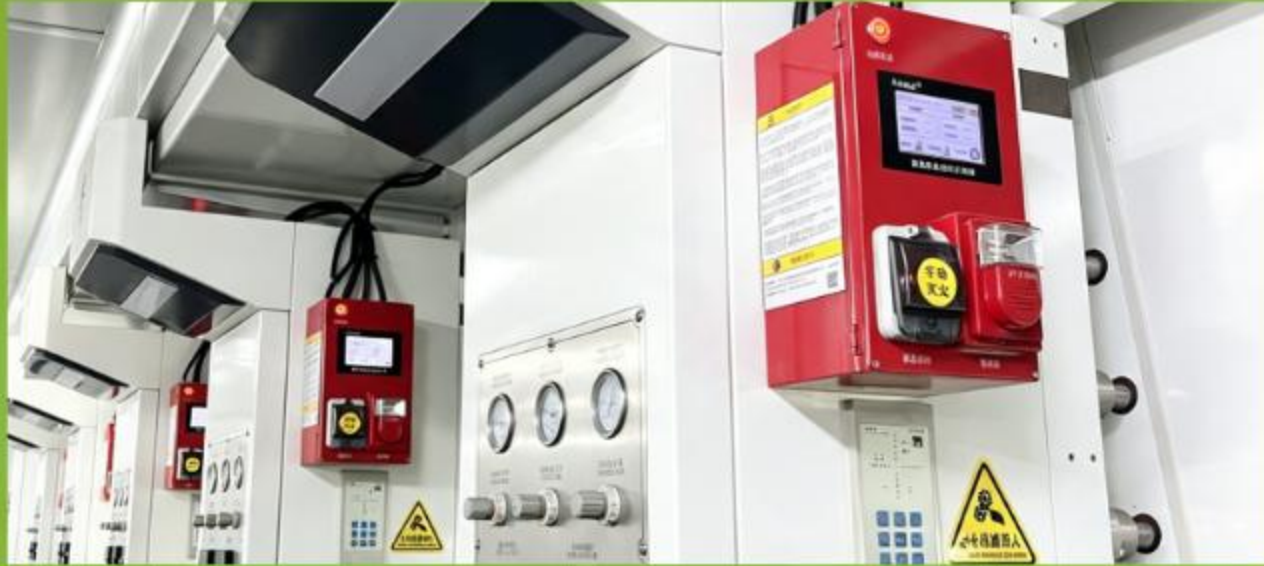
Automatic CO 2 fire-suppression system
